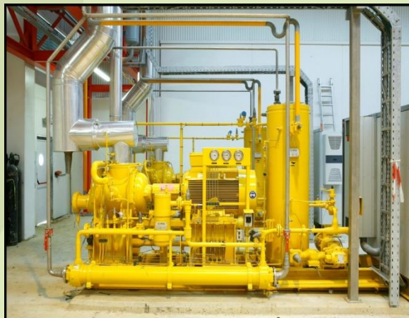
CO 2 recovery line
