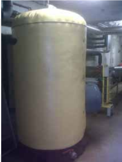
Storage tank for hot water
