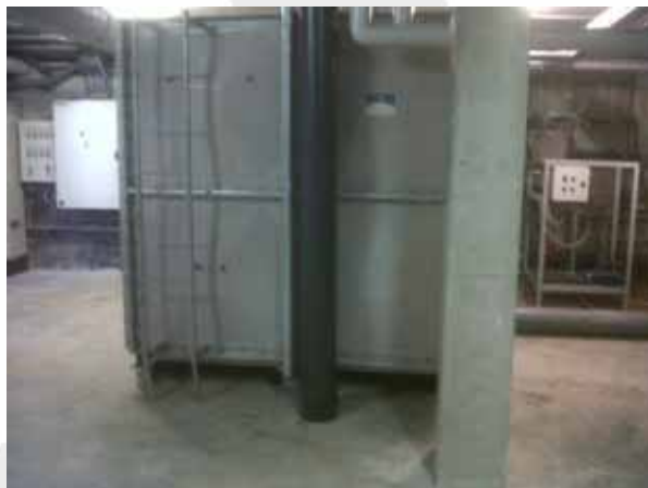
Buffer tank for reclaimed water
