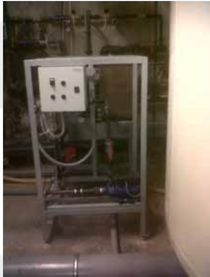
Exchanger system with pump and control
